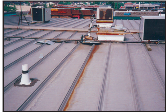
Example of corrosion caused by drainage from copper coils inside air conditioning units.
